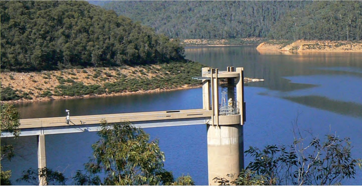
Corin Dam was completed in 1968 as the highest dam up the Cotter River. Photos: Matthew Higgins
